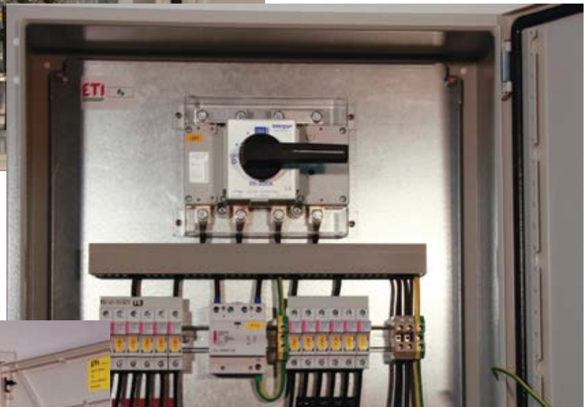
DC junction box (CH gPV fuses)
