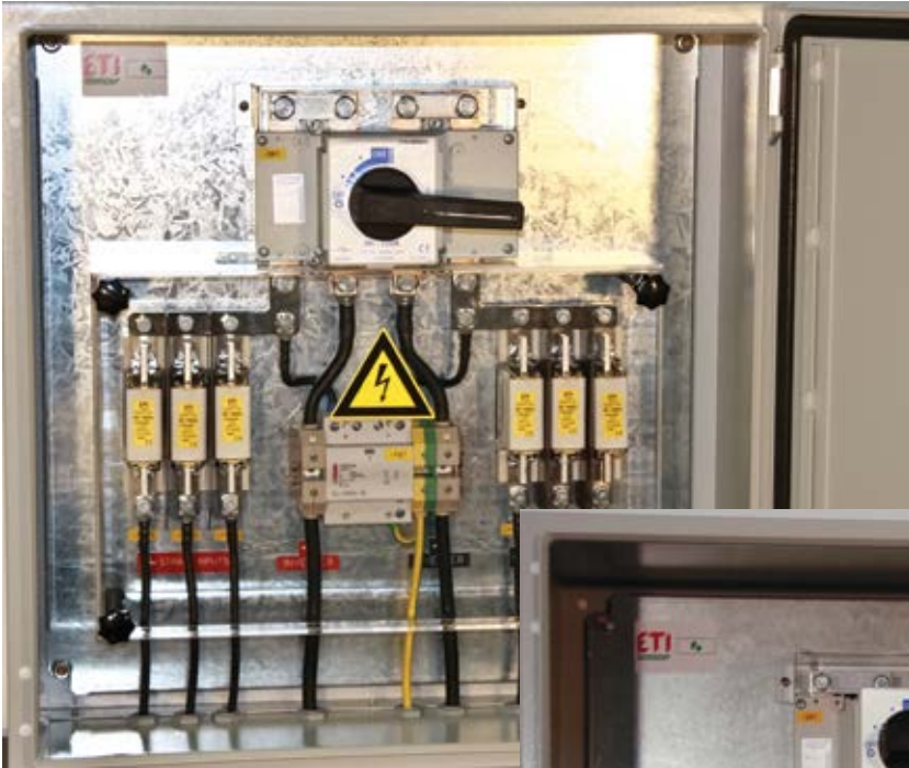
DC junction box (NH gPV fuses)
