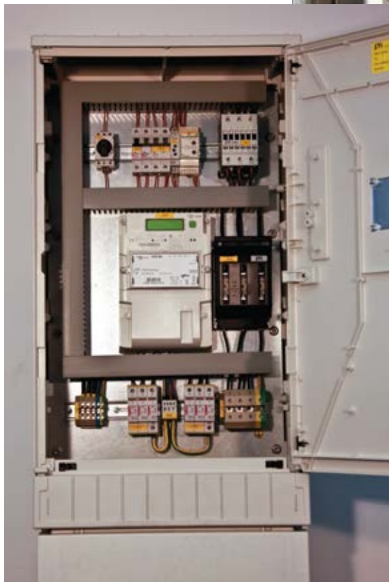
Meter distribution cabinet
